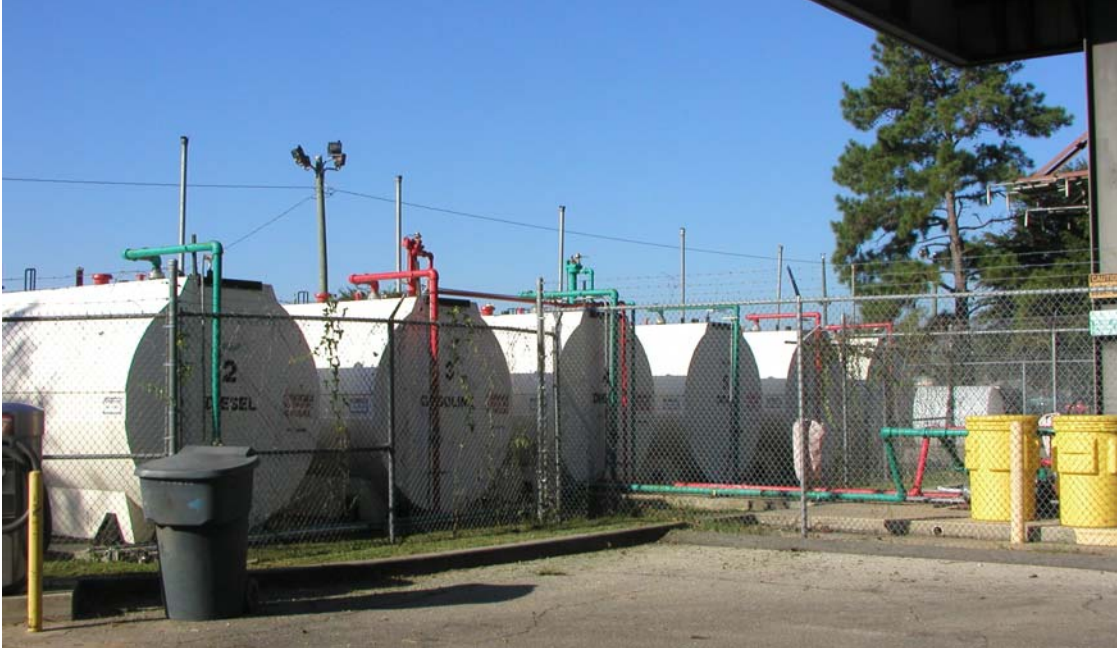
Large fuel tanks at a main facility
