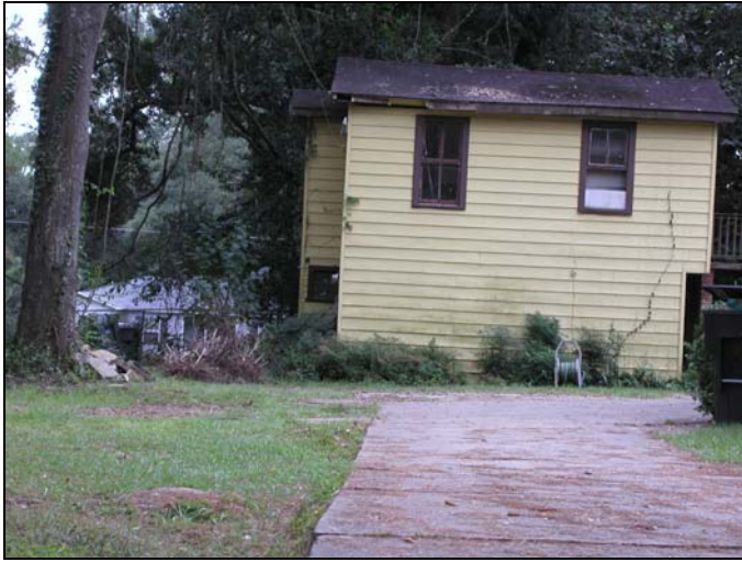
Case 4 – Before – 507 Gore – In October 2003, the windows and the eave of the roof needed repair. Weeds and shrubs were overgrown on the side of the building, with a vine growing up the wall. No screens were on the windows.
