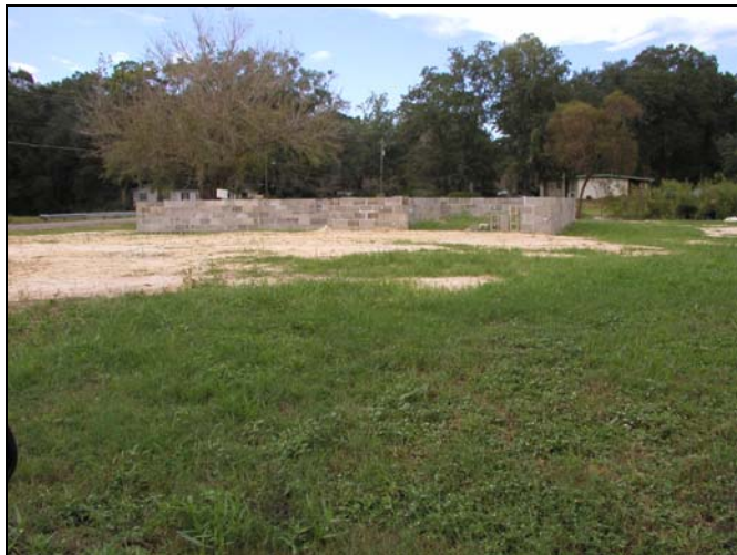
Case 6 – Before – 3301 Sunnyside – In October 2003, the foundation of a building was present, lot was mowed, and building materials were not present.
