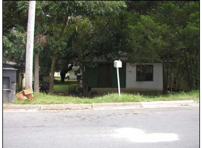
Case 5 – Before – 1213 Richmond – In October 2003, the front porch of the house needed repairs and the side stairs needed to be replaced.
