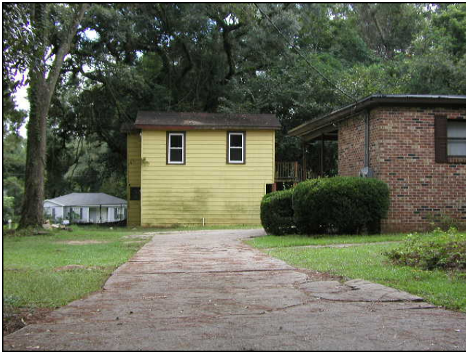
Case 4 – After – 507 Gore – In August 2004, new windows and screens had been installed, the roof eave repaired, and the weeds, vines, and shrubs removed.
